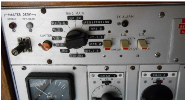
Figure 4. Pre-fade PPM and Ring Main switch
