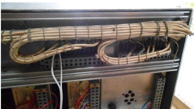
Figure 6. Original wiring loom
