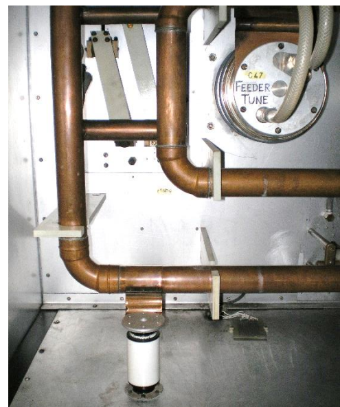
Figure 2. 54 mm copper pipes with elbows were configured as water-cooled inductors in the B6124
