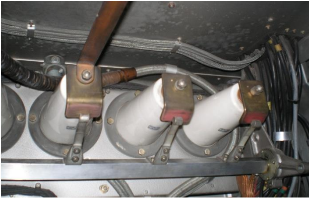
Figure 8. The pillar and earthing assembly inside the BD272 sender
