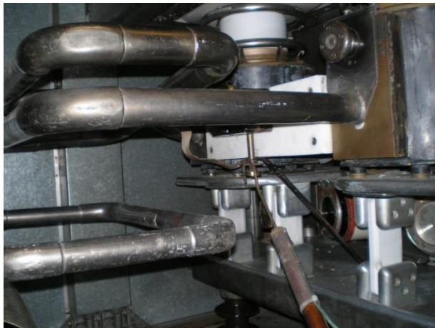
Figure 11. An earthing wand in use on the centre tap connection of the 11 kV modulated feed to the final RF amplifier in a BD272 sender
