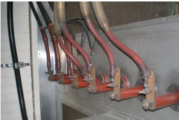
Figure 10. Substantial connection terminals near to the earthing mechanism
