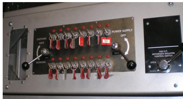
Figure 7. Isolation and earthing switches, together with the access keys, for the BD272 transmitter
