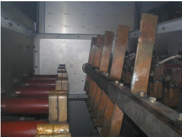
Figure 9. Earthing switch implementation as used on a B6124 300 kW sender
