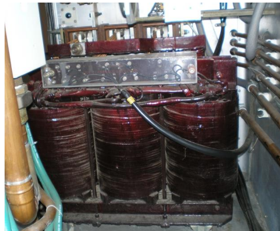
Figure 6. Filament transformer with Perspex shield
