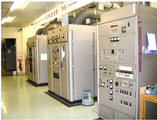
General view of a BD272 installation showing, left to right, modulator, RF and H1100 driver cubicles
